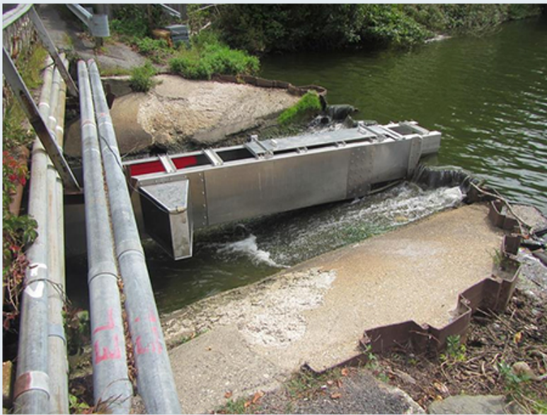
The fishway at Beaver Lake allows fish to pass underneath a bridge from Mill Neck Creek and Oyster Bay into Beaver Lake and freshwater habitat. A concrete spillway under the bridge, and the dam had blocked passage to the lake.
